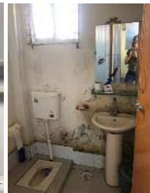
Toilet (less maintained)
