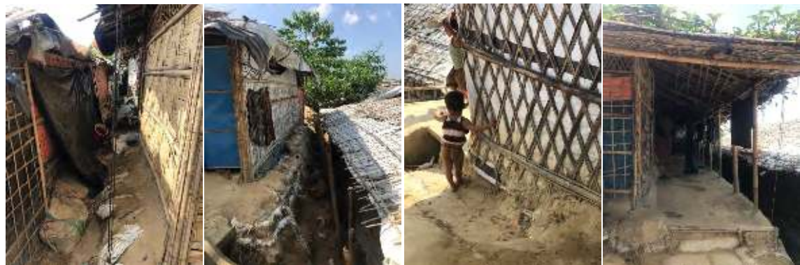
Inadequate drainage and lack of soil consolidation
