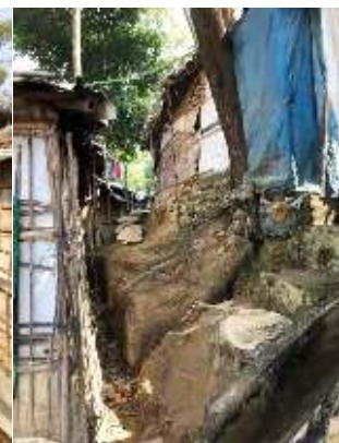
Lack of slope consolidation
