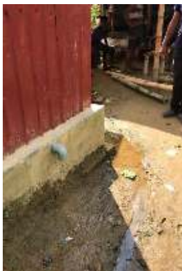
No proper drainage
