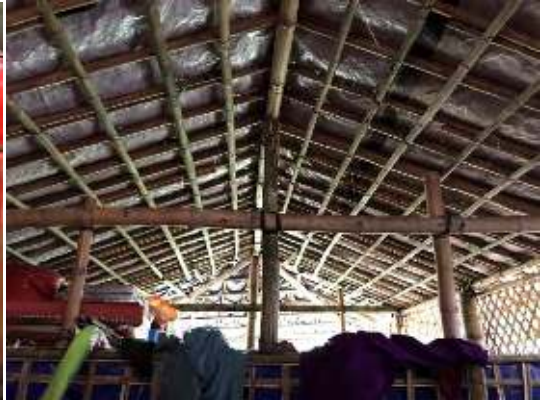
Big shelter: structure lacks essential material
